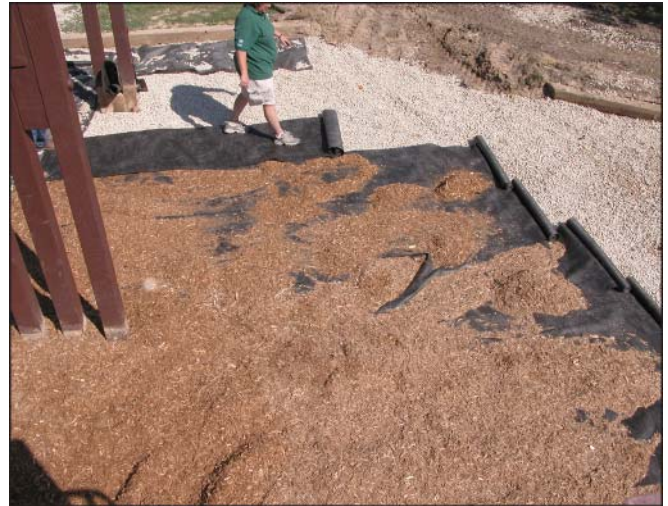
Figure 4—Completion of drainage system; second layer of fabric laid over drainage rock.
