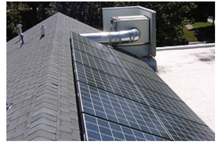
A solar array provides power for the Coolerado air conditioner, and the cool exhaust stream from the Coolerado improves the performance of the solar panels. (Photo by Coolerado)
