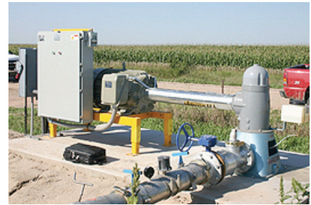
For agriculture and industry, the written pole motor offers a cleaner, more efficient alternative to fossil fuel-powered pumps. Precise Power will be demonstrating its written pole model at the DSM Motors and VFD workshop. (Photo by NPPD)
