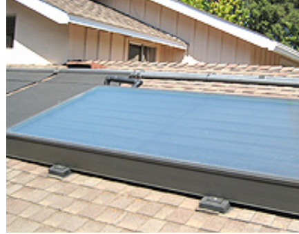
This is one of the first solar water heater systems to be installed under CPAU's new rebate program. Each installation must be inspected before the contractor can receive the rebate check. (Photo by California Center for Sustainable Energy)
