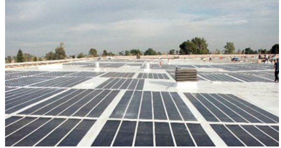
The Luke Air Force Base Exchange Building now boasts the Air Force's largest integrated photovoltaic roof system, thanks to an energy savings performance contract. (Photo by Luke Air Force Base)
