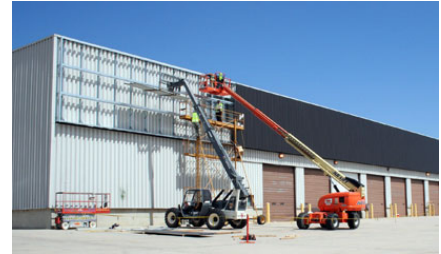
The SolarWall panels Fort Carson installed on a vehicle maintenance building improve ventilation and save energy costs. (Photo by Fort Carson)
