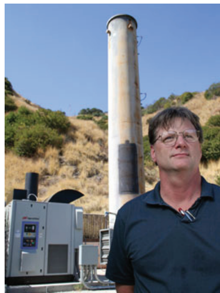
Combustion Turbine Specialist Rick Owen with Burbank Water and Power’s new 250-kW Ingersoll-Rand microturbine. (Photo by Burbank Water and Power)
