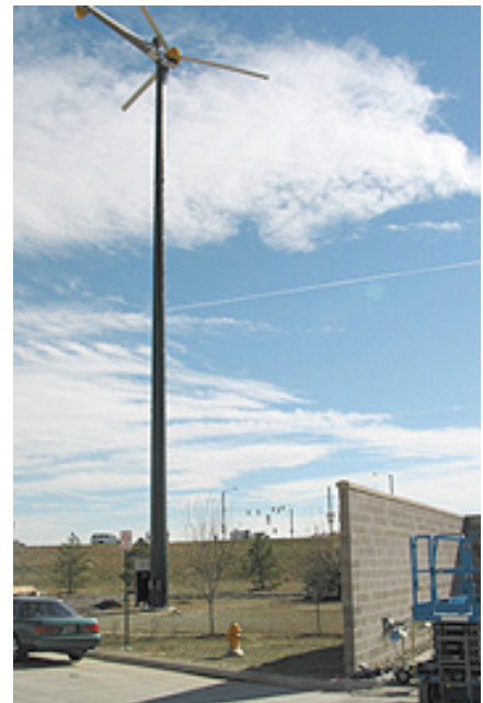
A 50-kW wind turbine is one of 50 sustainable measures being tested at Wal-Mart’s SuperCenter in Aurora, Colo.
