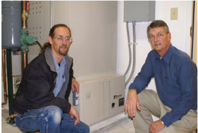
MPEI’s Master Electrician Guy Larson (left) and Member Services and Marketing Manager Gary Ashby inspect an installation of a Steffes ETS hydronic heating system. (Photo by Rob Taylor)
