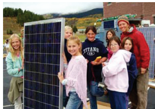
SEI Instructor Carol Weis teaches 5th graders how to check the charge on each solar panel before installing them. (Photo by Solar Energy International)
