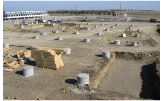
Construction is underway on four recovered energy powerplants along the Northern Border gas pipeline running through North and South Dakota. (Photo by Basin Electric Power Cooperative)
