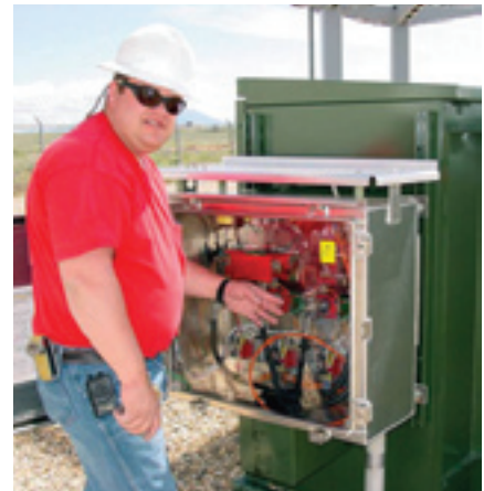
Meter Technician Bill Dahlke installs the substation equipment necessary to operate the Two Way Automatic Communications System. (Photo courtesy of Carbon Power & Light)
