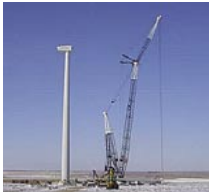
Contractors install the blades on Lamar's first wind turbine. The city commissioned the 1.5-MW unit on Feb. 27. (Photo courtesy of Lamar Light and Power)
