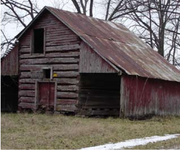
A barn at the Kofal Farm on the Mark Twain National Forest. The farm has been determined eligible for the National Register.
