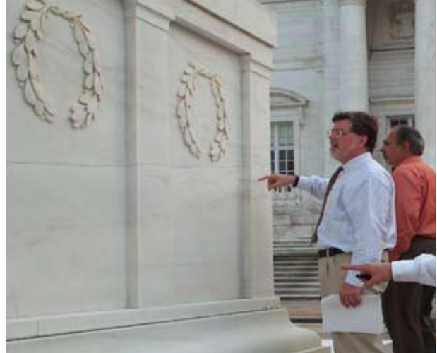
Site inspectors view the condition of a crack in the Tomb of the Unknowns Monument. (Photo courtesy U.S. Army Corps of Engineers, Baltimore District)
