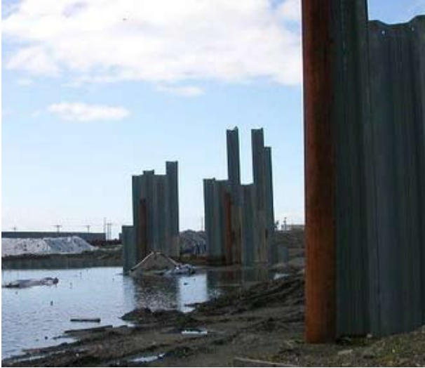
Halted work on the Port Angeles Graving Dock showing part of the area impacted by construction activities
