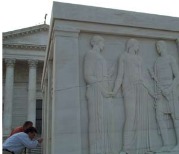
Cracks to the Tomb Monument and proposed replacement have caused concern in a number of groups due to the Tomb's historic status. (Photo courtesy U.S. Army Corps of Engineers, Baltimore District)
