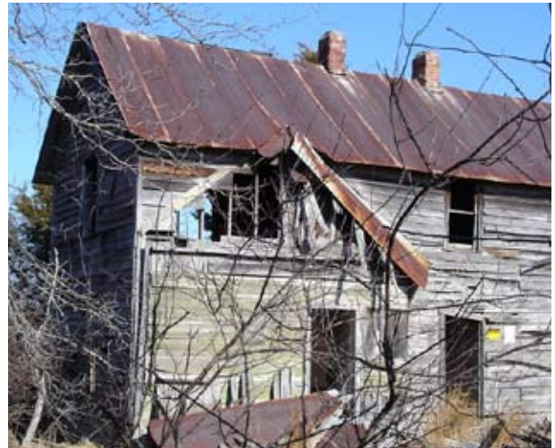
Bussman Farm on the Mark Twain National Forest has been determined eligible for the National Register and is proposed for demolition.
