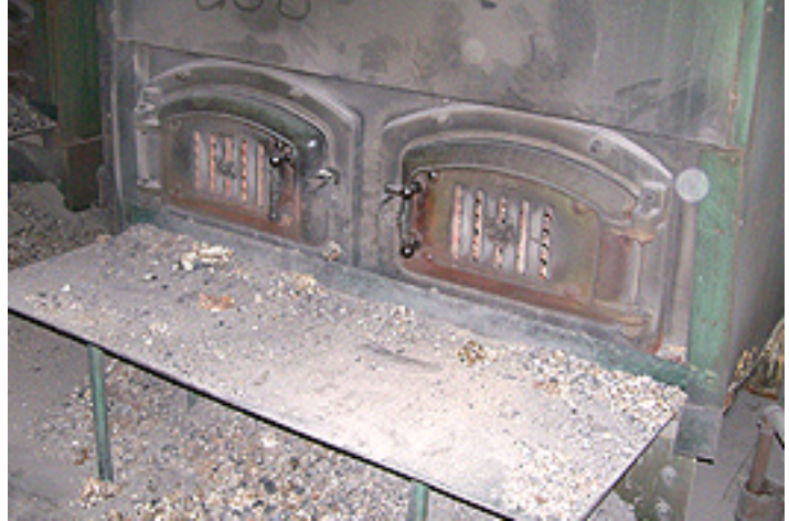
This old coal boiler was one of the last in operation in a Colorado school district. The new heating system includes a wood chip boiler and geothermal heat pumps. (Photo by McKinstry)
