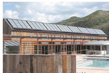
The Community Office for Resource Efficiency gave Snowmass Village, Colo., a $40k grant to install a solar water heating system on the town’s recreation center. The city of Aspen’s Renewable Energy Mitigation Program funds CORE programs. (Photo by Community Office of Resource Efficiency)
