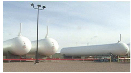
These tanks are part of the propane-air mix plant that Ellsworth installed under its utility energy services contract with Montana-Dakota Utilities Co. UESCs help Federal facilities finance large-scale energy efficiency improvements. (Photo by Ellsworth Air Force Base)
