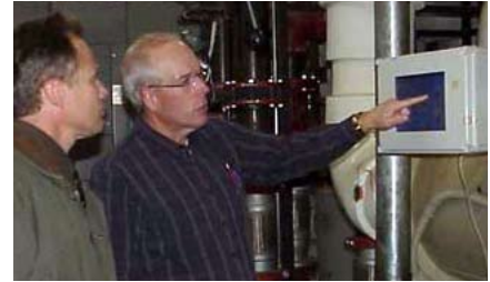
Project Engineer Rich Ivey, right, shows Energy Services Representative Greg Vaselaar the touch-screen controls on the new chiller in the South Dakota capitol building. (Photo by Michele Farris)
