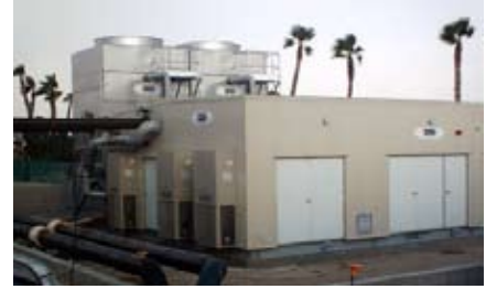
A modular chiller plant replaced 25 rooftop air conditioning units on the Avi Resort and Casino, reducing the energy costs and allowing for future facility expansions. (Photo by TAS)
