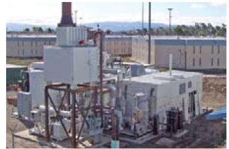
This 1-MW hydrogen fuel cell supplies 50 percent of the electricity for the Santa Rita Jail in Alameda County, Calif. With a 1.2-MW solar array on its rooftop, the jail generates up to 80 percent of its electricity from onsite ultraclean and renewable resources. (Photo by Alameda County)
