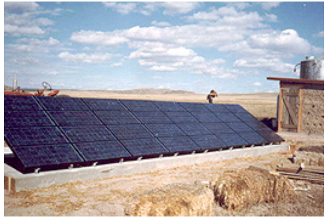
The irrigation system at Wolfberry Farm in Arizona’s Chino Valley runs off the power generated by 32 40-watt solar panels. (Photo by Tim Crews)
