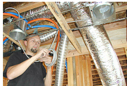
An electrical technician installs a CKP62 high-output CFL downlighting system at a field test site in Sacramento, Calif. Title 24 updates encourage this kind of high-efficacy lighting in rooms with high loads and long use hours. (Photo by California Lighting Technology Center )
