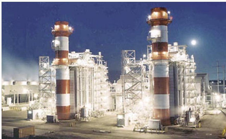
The 533-MW, combined cycle Valley Generating Station is among 10 natural gas-fired powerplants LADWP is "repowering" as part of its IRP. (Photo courtesy of Los Angeles Department of Water and Power)
