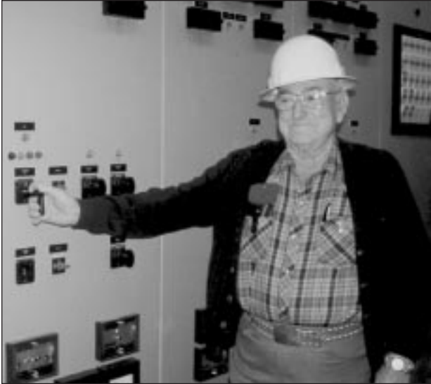
Former Valley Electric Association board member Oakie Spears throws the switch to energize the 230-kV line.
