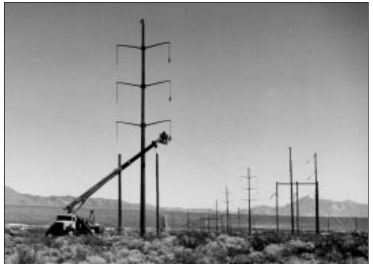
Construction takes place near Pahrump, Nev., on Valley Electric Association's 230-kV transmission line which connects to Western's Mead Substation.
