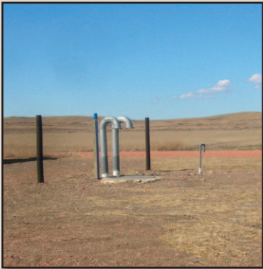
Typical Water Pipeline Vent
