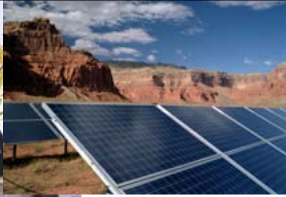
PV solar arrays for larger-scale electricity.
