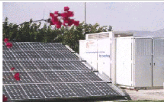
Hydrogen production by photovoltaic hydrolysis.
