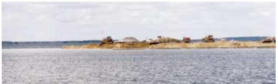
Figure 2. Rebuilding North Dakota State Highway 57, which was flooded by Devils Lake. (Photograph by the North Dakota Department of Transportation.)
