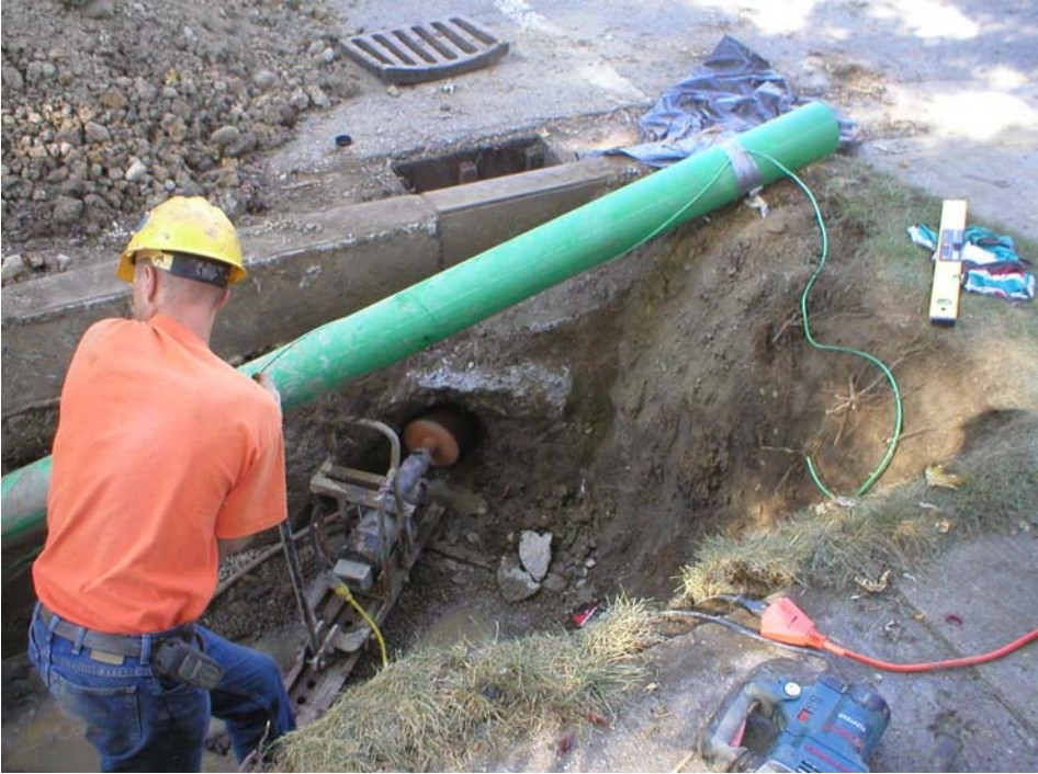
Figure 8-5. Curb drains convey disconnected footing drain flow to the storm water system.
