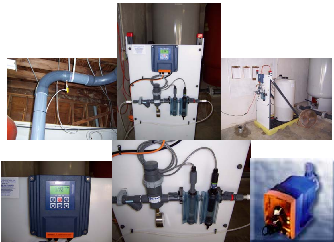
Figure 4-6. Chlorine Injection System
