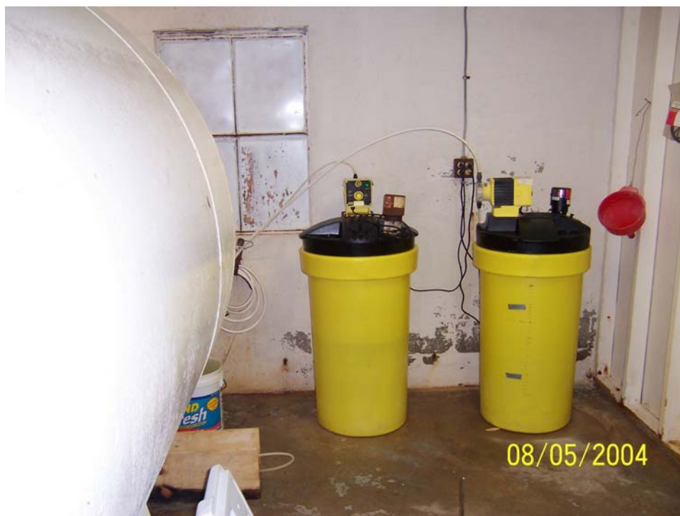
Figure 4-2. Preexisting Chlorine and Polyphosphate Addition Systems
