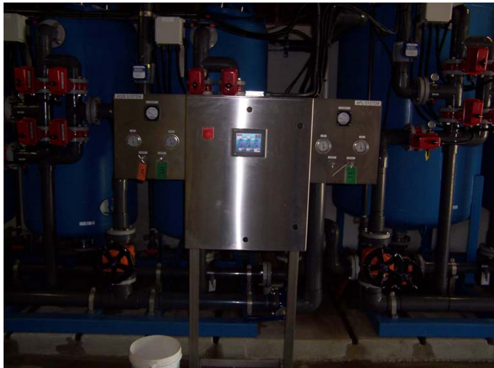
Figure 4-10. System Control Panel
