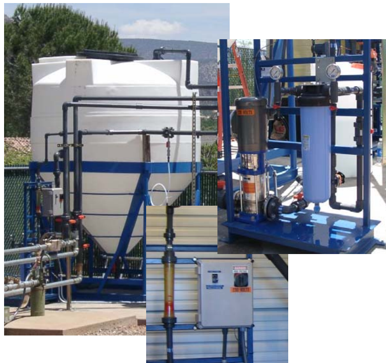
Figure 4-6. Backwash Process Components (Clockwise from Left: 1,800-gal Holding Tank; Recycle Pump and Bag Filter; and Backwash Flowrate Indicator and Pump Box)
