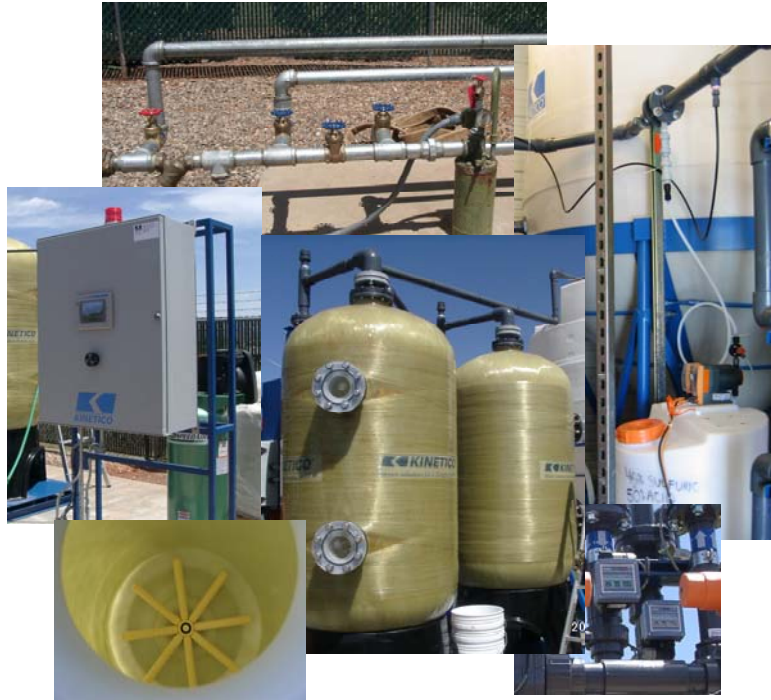
Figure 4-5. Treatment Process Components (Clockwise from Top: POE Well No. 2 and Treatment System Bypass Piping; Acid Addition Setup; In-Line pH Meter; Adsorption Tanks and Lower Distributor; and Main Control Panel)
