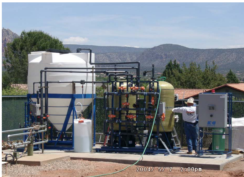
Figure 4-4. Kinetico's FA-236-AS Treatment System on Concrete Pad
