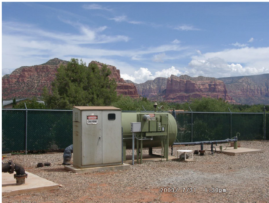
Figure 4-1. Predemonstration Site Conditions (Right to Left: Wellhead, Piping, Hydropneumatic Tank, Electrical Panel, and Chlorine Shed)
