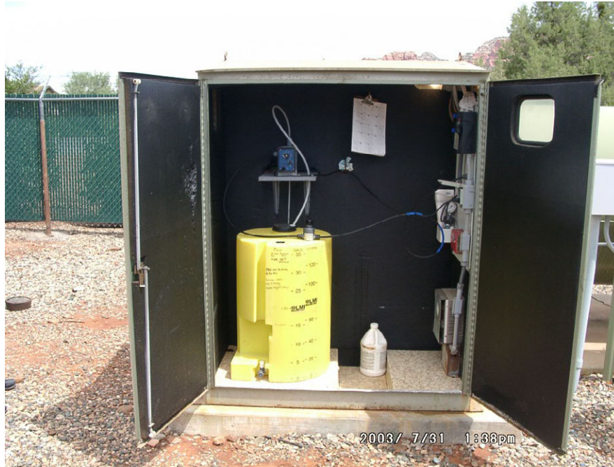
Figure 4-2. Existing Chlorine Injection System
