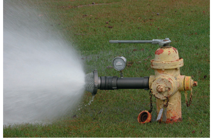
Figure 4-6. A Hydrant Being Flowed with a Diffuser as Part of a Fire-Flow Test.
