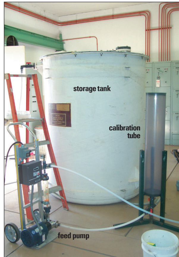
Figure 3-3. Tracer Injection Setup (Storage Tank, Calibration Tube and Feed Pump).
