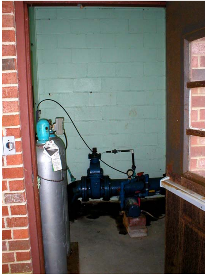
Figure 4-2. Chlorine Gas System at Well No. 1
