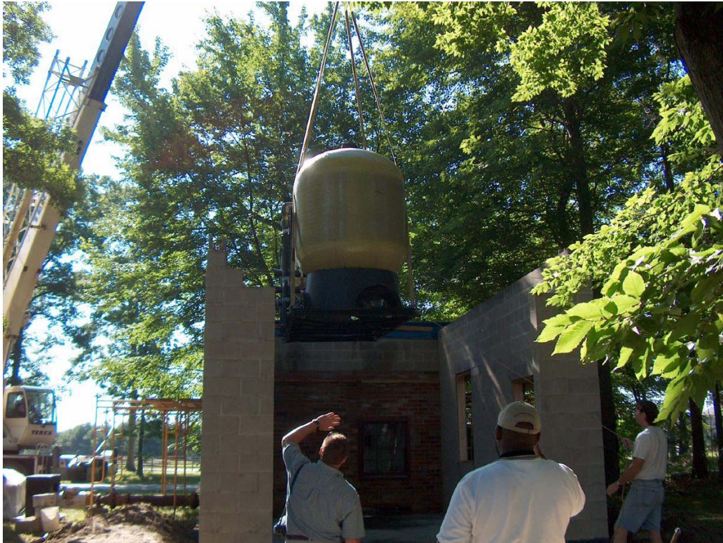
Figure 4-6. Unloading of the APU Skid into the Partially Completed Treatment Building Addition
