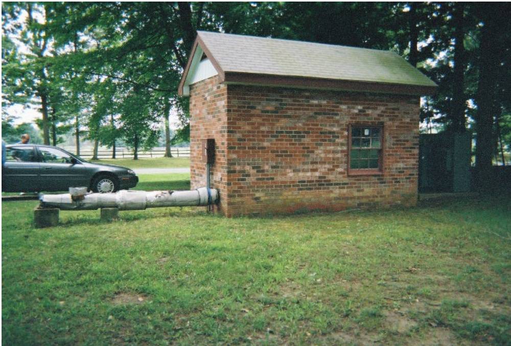
Figure 4-1. Existing Well House No. 1
