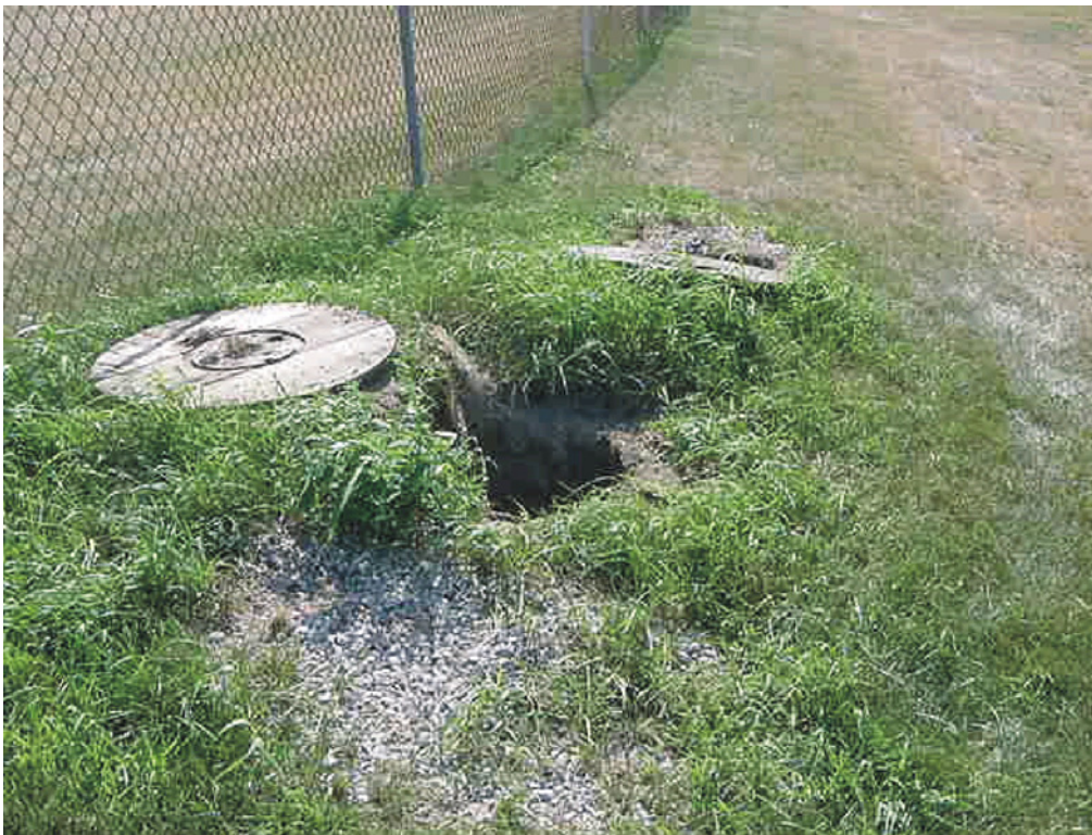
Abandoned Hole for Baseball Field Lighting Installation
