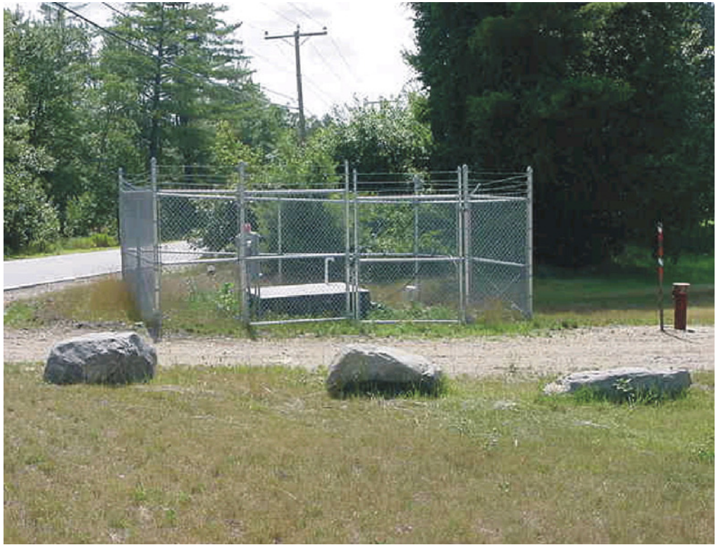
Infiltration Pumping System on the Somersworth Site
