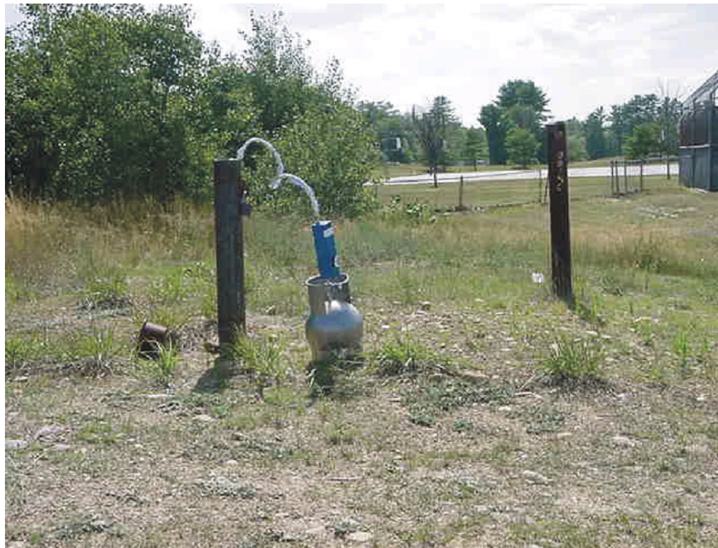
Sampling a Somersworth Landfill Gas Well
