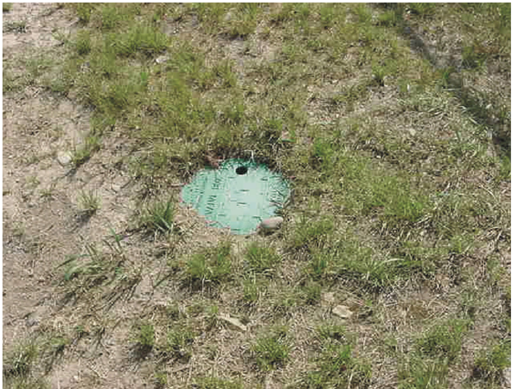
Valve Box near the Baseball Field at the Site Entrance
