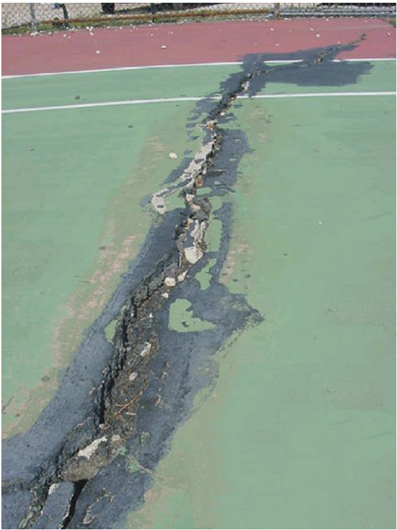
Cracks in the Tennis Court Surface
