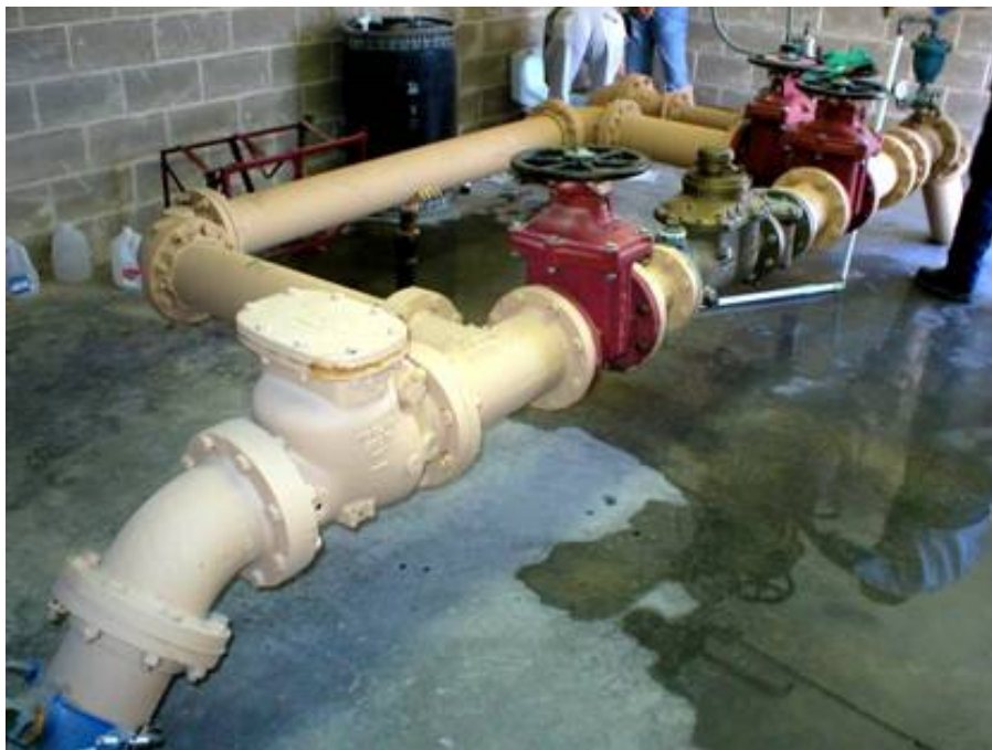
Figure 4-3. Piping Inside the Pump House at the Desert Sands MDWCA Site
