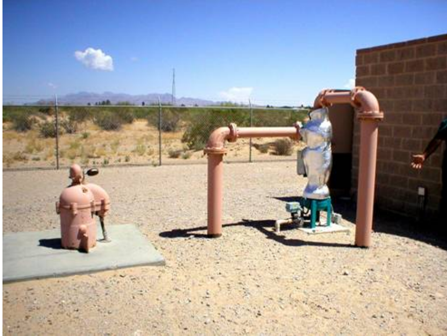
Figure 4-2. Well No. 3 (Left) and In-Line Sand Separator (Center) Adjacent to the Pump House (Right) at the Desert Sands MDWCA Site
