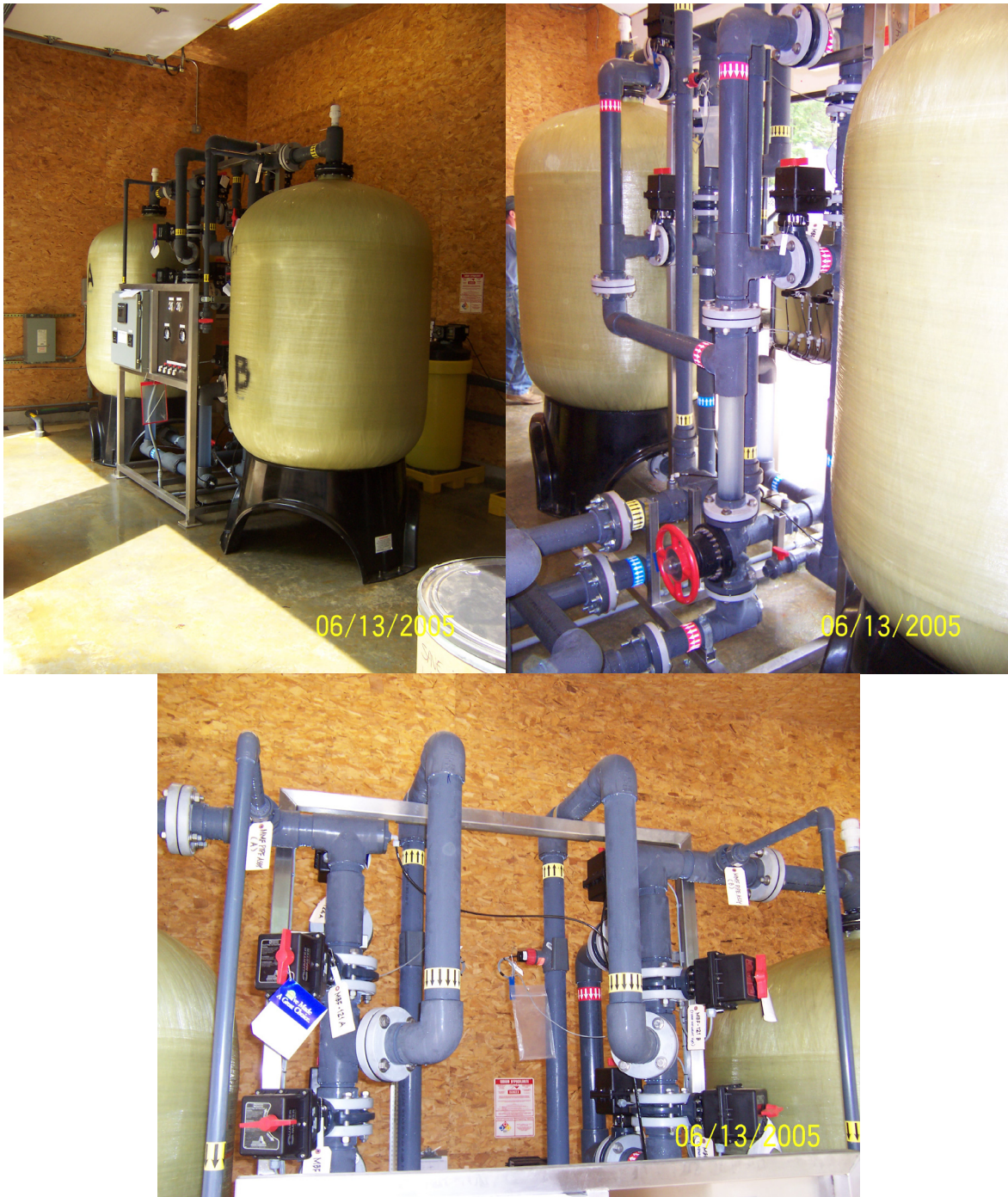
Figure 4-7. APU-RWS Treatment System (top left) with Valve Tree (bottom) and Backside of System Piping Including Backwash Sight Glass (top right)
