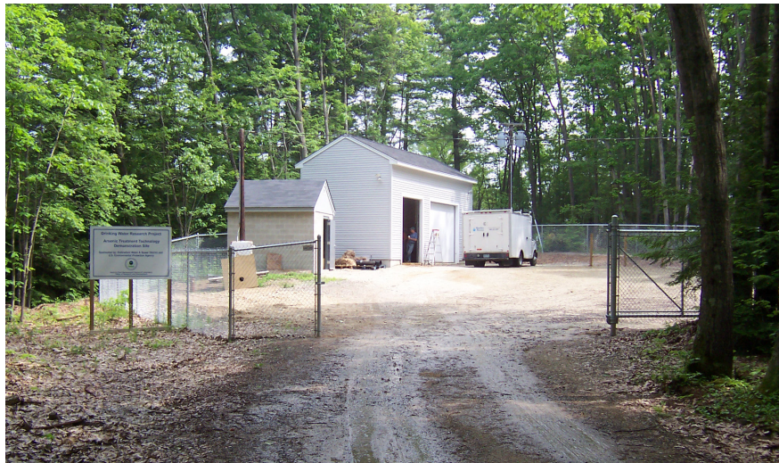
Figure 4-8. Porter Well House Area after Building Construction and Treatment System Installation ( Large Treatment Building Addition in Background, Fenced Parking Area, and EPA Demonstration Project Sign to left of Gated Entrance )
