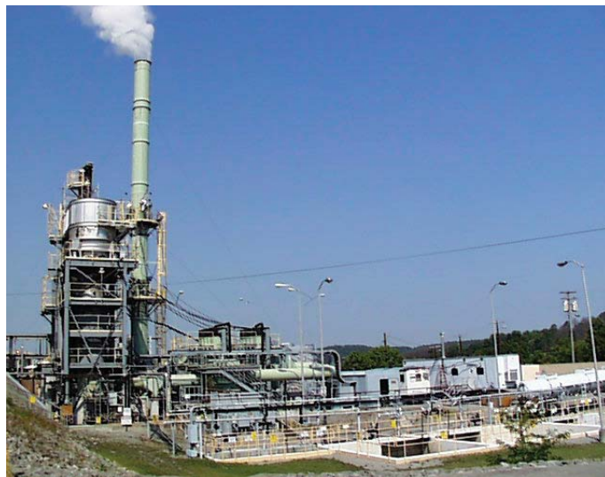
One of the test locations for mercury CEM verification
