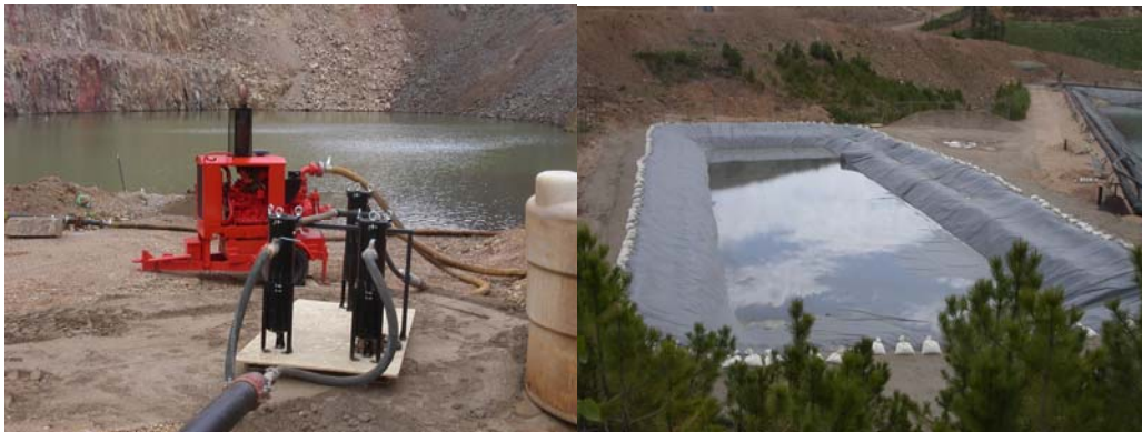
Figure B-1. (left) Godwin pump and filter-set configuration in the pit; (right) aeration/settling lagoon (ASL) with initial 2,000 gallon run
