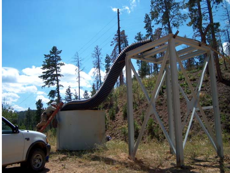
Figure B-4. “Riffle run” for aerating ASL water prior to discharge; the discharge line connects to the fitting on lower tank, connecting with a tributary clean water-diversion pipe near the base of slope.
