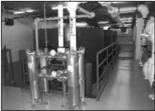
Rainwater collection system saves an estimated 1.4 million gallons of water each year.
