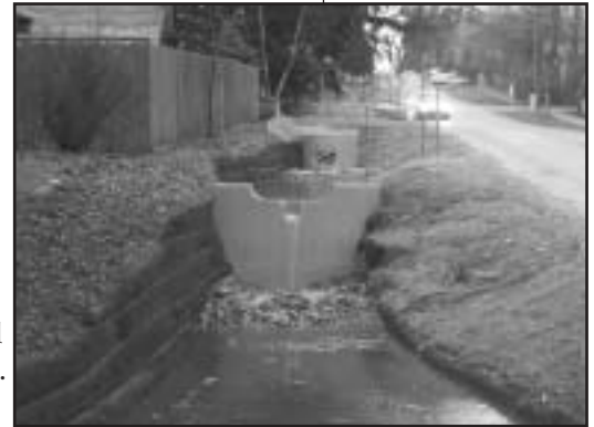
The Cascade Prototype project at N. 110th St. after most of the construction has been completed and before planting.
