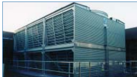
By increasing the efficiency of its cooling tower, ESC has saved both water and money.
