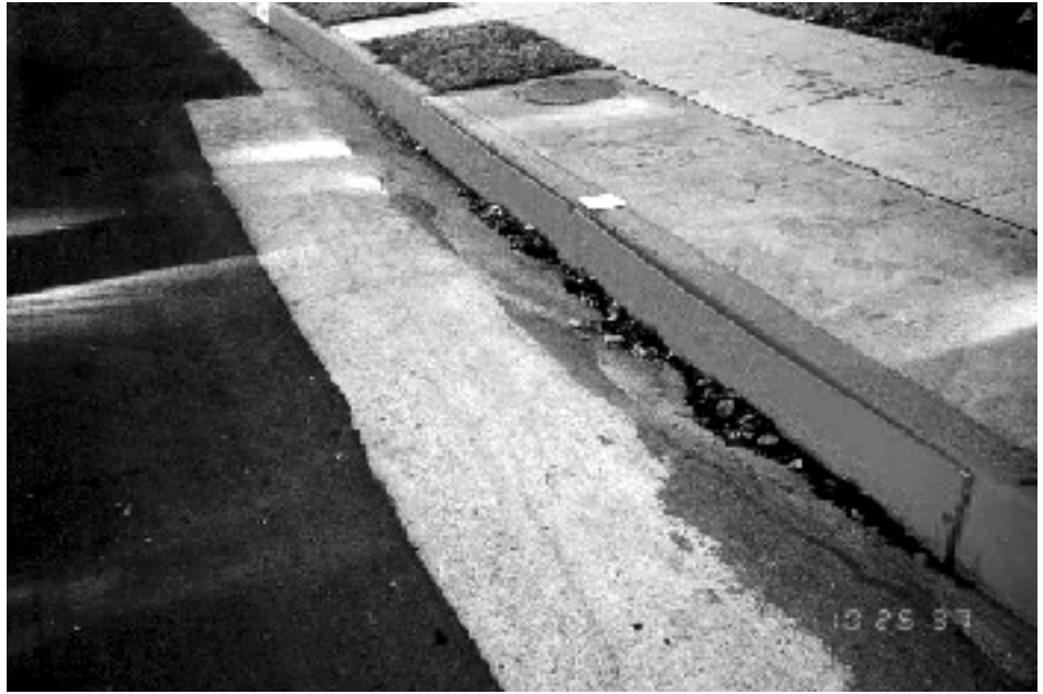
A "boardover" used to physically block the curb inlet of the catchbasin
