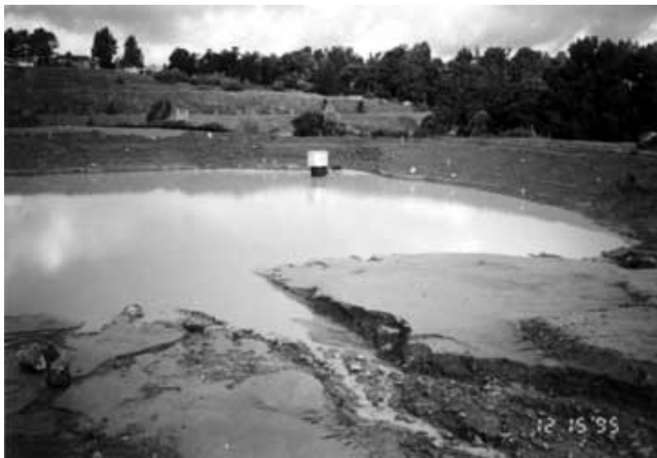
An improperly sized sediment basin is likely to fail in a storm event.
