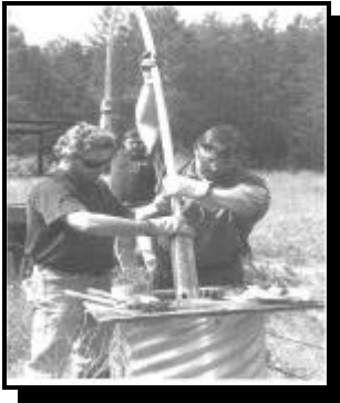
Figure 5: SRS monitoring well. (Source: SRS Environmental Report for 2000, Summary)
