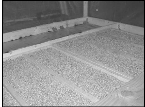
Figure 27: Interior of Artificial Attic of Main Containment - View from plywood floor looking at vermiculite in simulated trusses.
