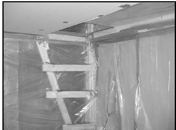
Figure 28: Interior of Artificial Living Space of Main Containment - View of drywall ceiling, plywood ceiling, and open access panel to attic.
