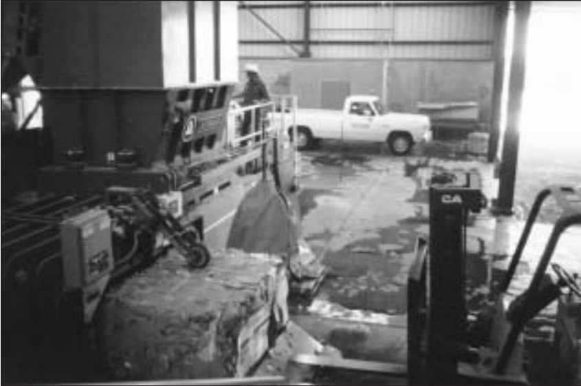
Solid waste baler compacts waste into dense, self-contained bales.
