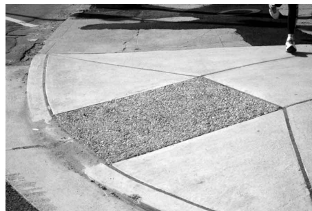
FIG. 5-2. CURB RAMP EXPOSED AGGREGATE SURFACE IN VIRGINIA. PEDESTRIANS WHO ARE BLIND DO NOT RELIABLY DETECT EXPOSED AGGREGATE CONCRETE.
