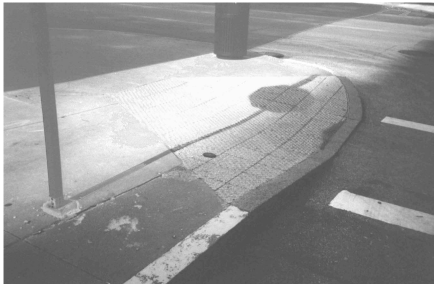
FIG. 5-13. TRUNCATED DOME PAVERS CUT AND FITTED TO THE ENTIRE SURFACE OF A PERPEN- DICULAR CURB RAMP, INCLUDING FLARES, CLEVELAND, OH.
