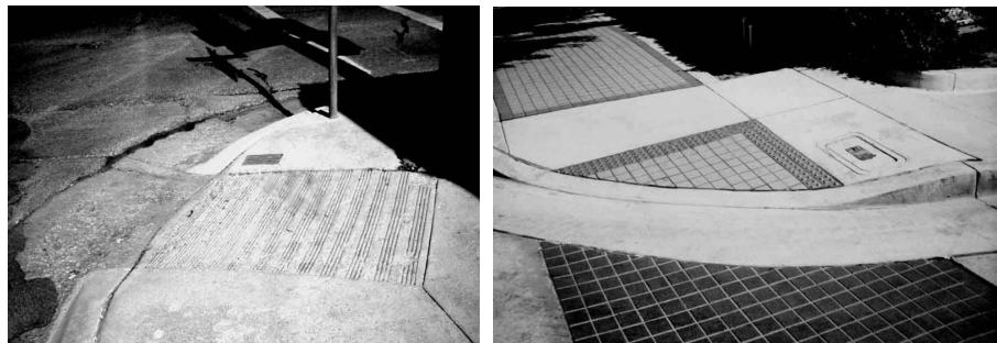
FIG. 1-4. (LEFT) CURB RAMP WITH A MINIMALLY DETECTABLE GROOVED SURFACE IN PHOENIX. FIG. 1-5 (RIGHT) A CURB RAMP WITH A NARROW BORDER OF DETECTABLE WARNING PAVERS AT THE SIDES AND SMOOTH PAVERS IN THE MIDDLE. BLIND PEDESTRIANS COULD EASILY MISS THE NARROW BORDER OF DETECTABLE WARNING PAVERS.
