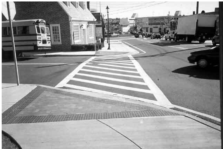
FIG. 5-14. A BAND OF DETECTABLE WARNING PAVERS OUTLINES THE TRIANGULAR SHAPE OF THIS CURB RAMP IN TOWSON, MD.
