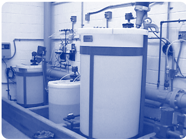
With a DWSRF loan, an aging water system in Braddock Heights was abandoned and replaced with a new system
