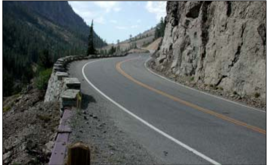
The portion of the East Entrance Road between Sylvan Pass and the East Entrance Gate will be reconstructed to a 30-foot width beginning in 2004.
