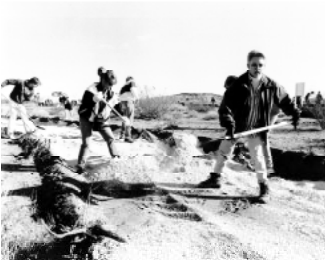
Volunteers build a trail adjacent to a wetlands in the new Boulder City, Nevada, Veterans Memorial Park. The wetlands is being created by Reclamation, City of Boulder City, and Nevada Department of Wildlife (photo by Reclamation).
