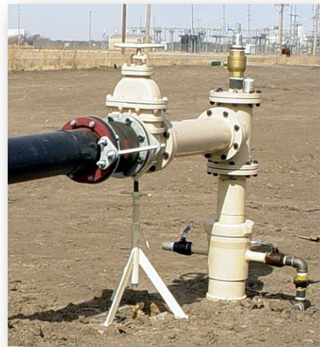
UIC Injection Well Head
