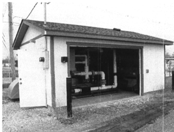
Figure 9 – Colorado Avenue Subsite – Phase III, 6th Avenue IWA System.
