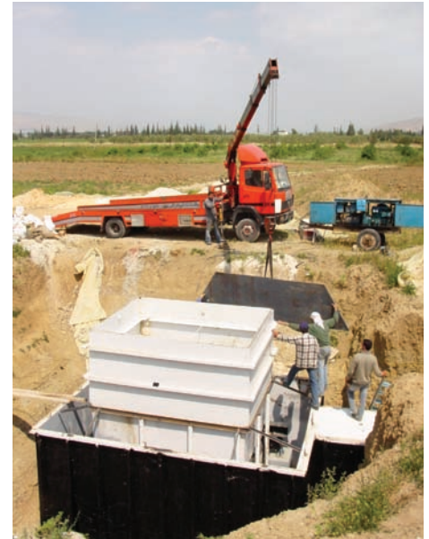
Construction of a large weighing lysimeter at the Dayr Alla Research Station of the Jordanian National Centre for Agricultural Research and Extension.
