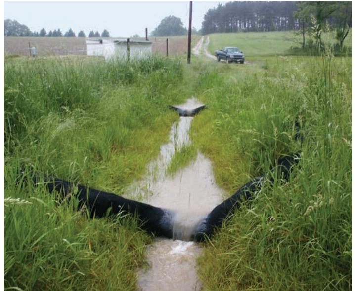
Runoff from a field planted with corn is directed into a grassed waterway where it passes through and over a series of compost-filled filter socks that help reduce levels of nutrients and herbicides.
