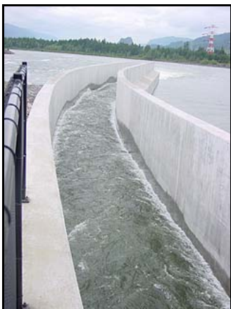
(B2 Corner Collector, photo by Corps)
