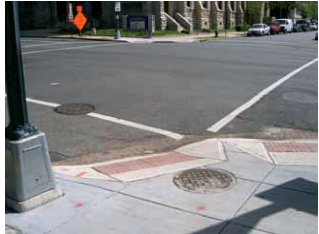
An urban intersection with paired perpendicular curb ramps, each with a 2-foot strip of detectable warnings at the toe. The flares have been shortened so that the ramps will both fit on the corner (flares are not a part of the pedestrian access route.)
