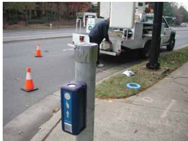
APS may need to be installed on a new stub pole at the departure curb for optimum usability.
