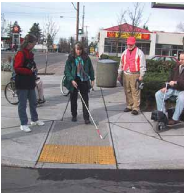
PROWAAC members observe a thin-film detectable warning retrofit on an existing curb ramp in a pilot project in Portland, OR
