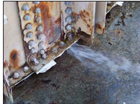
Leaking Campo Water Tank, Campo Band of Kumeyaay Nation, Campo, CA
