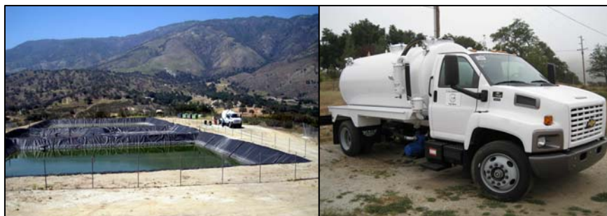
Left: Waste water lagoons; Right: La Jolla Septic Pump Truck; La Jolla Band of Luiseño Indians, Pauma Valley, CA
