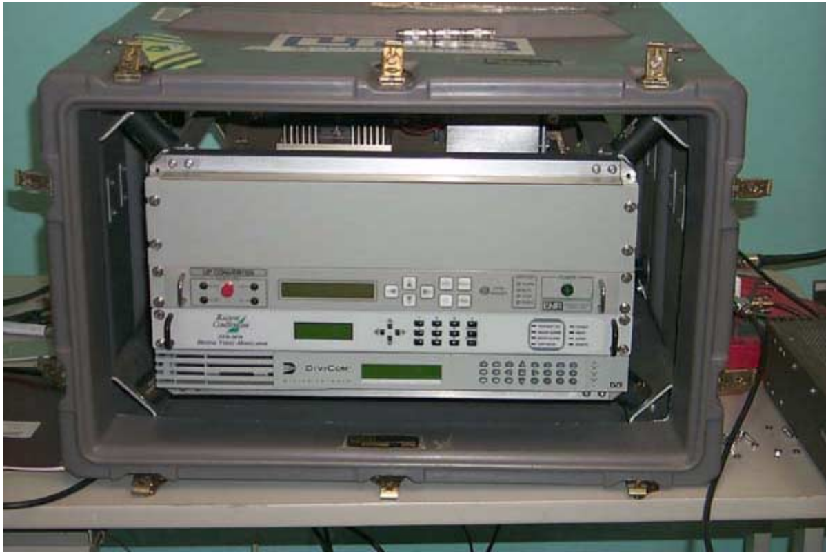
Figure A-5. Northpoint MVDDS Single Channel Transmitter
