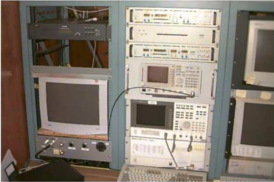
Photo F-3. Starboard Half of Equipment Rack Showing Signal Attenuator Panel, Data Collection Receivers, Vector Signal Analyzer, and Spectrum Analyzer
