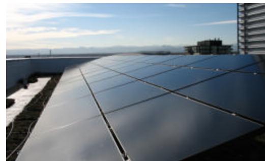
Solar panels were installed on the roof of EPA's Region 8 office in Denver, which achieved LEED Gold certification in 2007.
