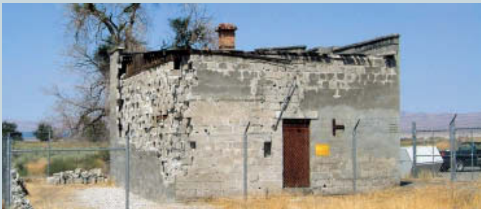
Work may begin this fall to restore the crumbling wall of the First Bank of White Bluffs, built in 1907. Scouts, students and other volunteers will mold more than 100 of the unusual E-shaped blocks as part of the restoration project. Volunteers and the staff of Hanford Reach National Monument, WA, hauled off old cedar roof shakes, disintegrated wall plaster and 60 years of bird guano as the first step in restoration. (Jenna Gaston/USFWS)
